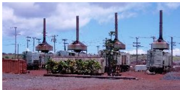
(6) 1.0 MW EMD Diesel Generators (2) 2.2 MW Caterpillar Diesel
