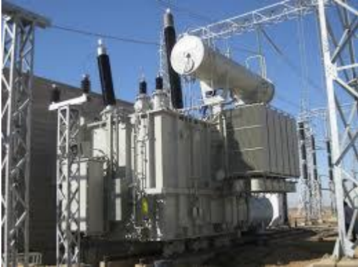
High Voltage Transformers
